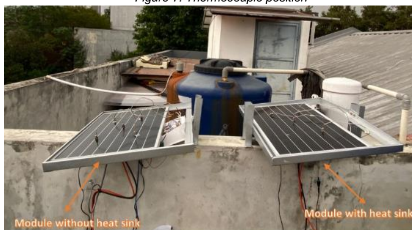
Figure 8. Solar panel with heatsink and without heatsink
