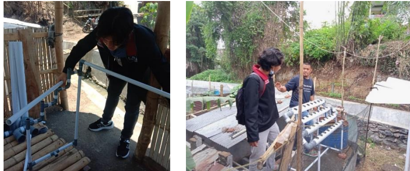
Figure 4. Hydroponic installation assembly
