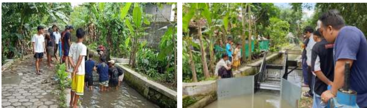
Figure 7. Submission of goods grants and installation of a mechanical bar screen device
