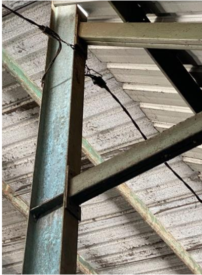
Figure 3. The corroded structural steel
