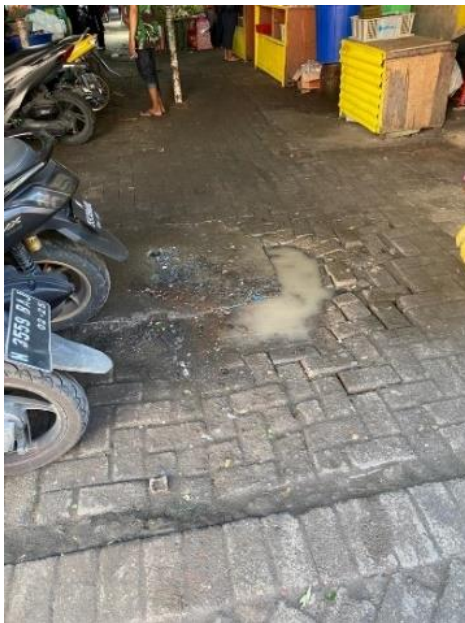
Figure 5. The sunken pavers at the market aisle
