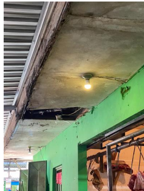
Figure 6. The damaged ceiling in market stalls
