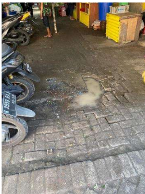
Figure 5. The sunken pavers at the market aisle
