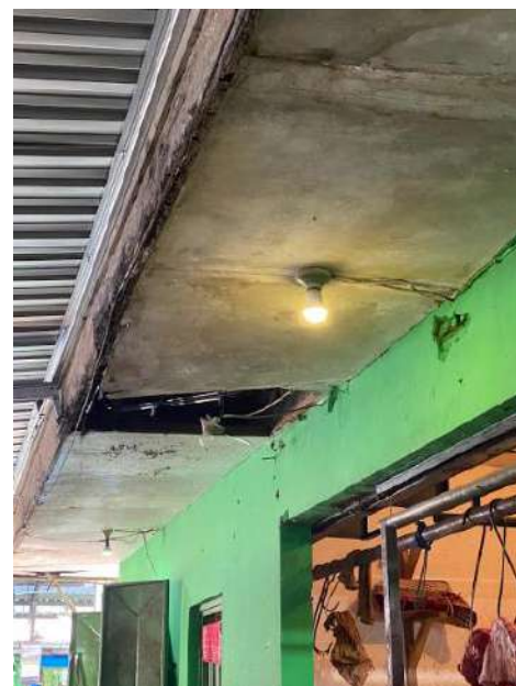
Figure 6. The damaged ceiling in market stalls
