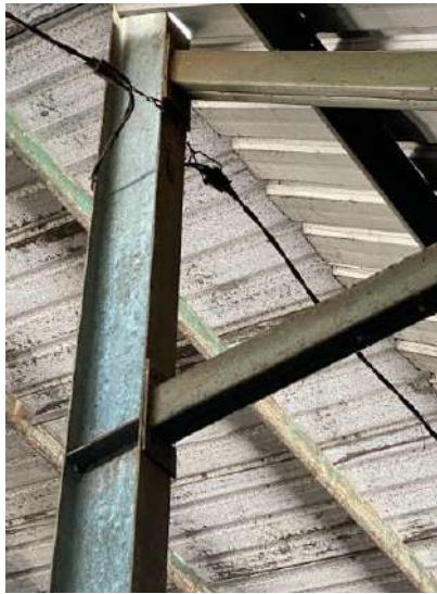
Figure 3. The corroded structural steel
