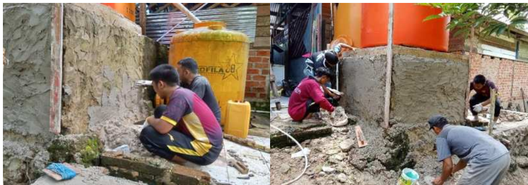
Figure 4. Rainwater harvesting equipment
